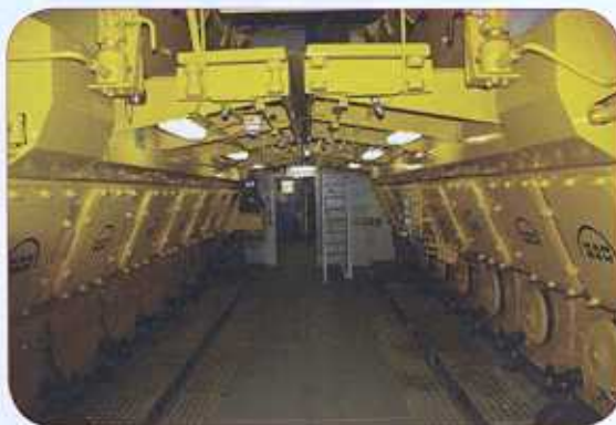
The Man B&W engines aboard the HAWAII are part of an incredibly vast engine room expertly attended to by MEBA officers.
